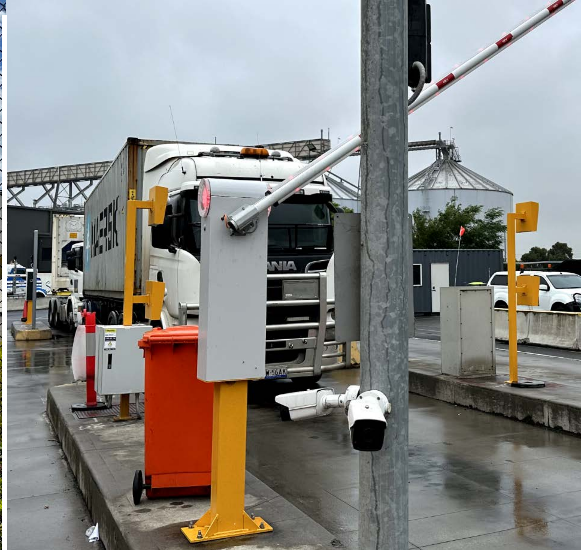
Vehicle lane with cameras for LPR and driver identification
